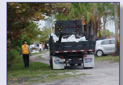
ICA crew collects bags of trash to be hauled to Dade Co. recycling and disposal facilities
