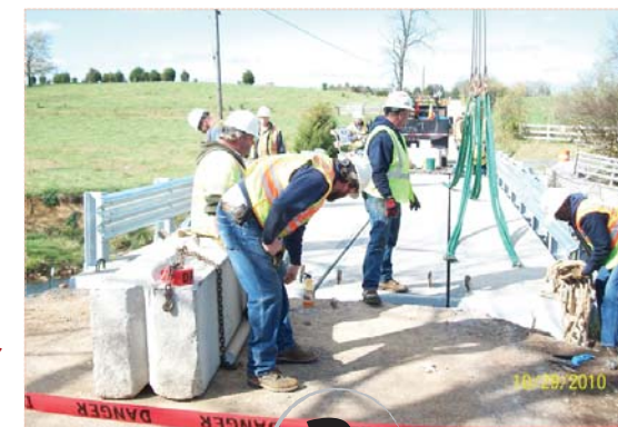
Another bridge in Virginia gets a makeover by the Virginia Design/Build Bridge crew
