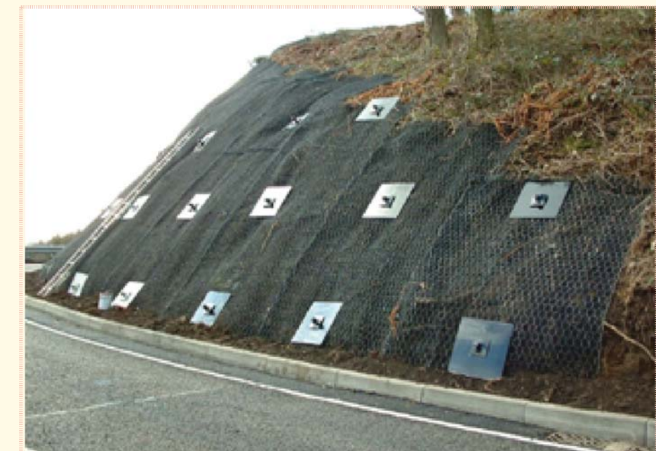
F&H will investigate and develop design solutions for embankment failures along a 1-mile stretch of US 421 for The Kentucky Transportation Cabinet.
