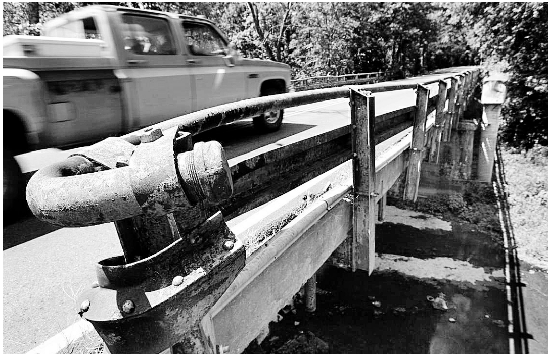
The West Harpeth River bridge on Southall Road was identified last year as structurally deficient but not unsafe for driving.
